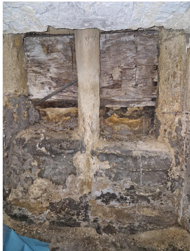
Figure 3 shows a boarded-up window in the cellars of the old schoolmaster's house (Author's own 2024).
